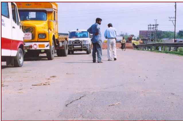
Bitumen cracks due to roadside ASM coal mining.
